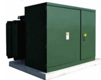
Aux. Transformer 6' (L) x 4.5' (W) x 5-6' (H)
