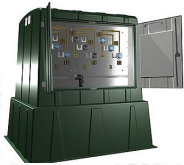
Switchgear 7' (L) x 7' (W) x 5-7' (H)
