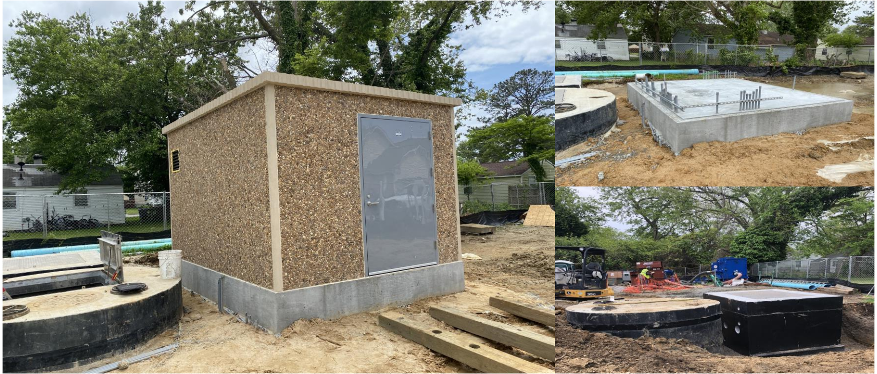
Replacement of the wastewater pump station in the North King Street Neighborhood
