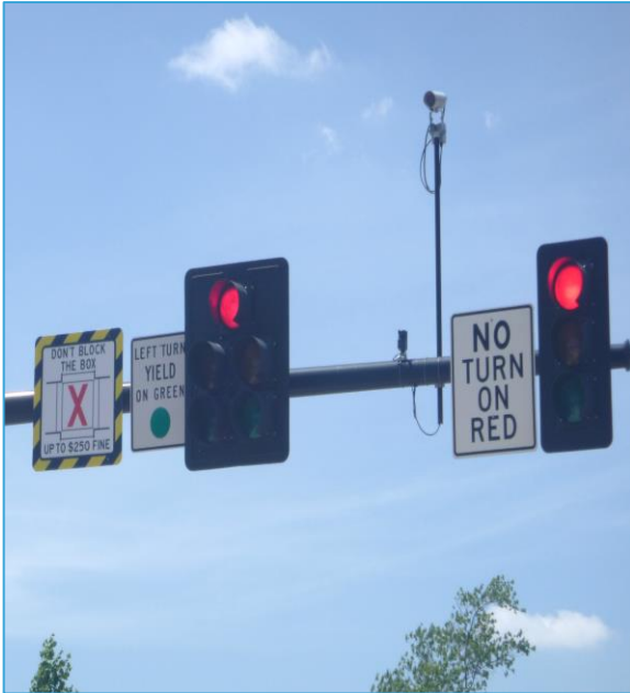
New LED street lights, traffic signs, and vehicle detection systems
